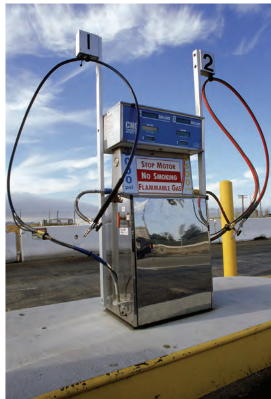
Compressed Natural Gas Dispensing
